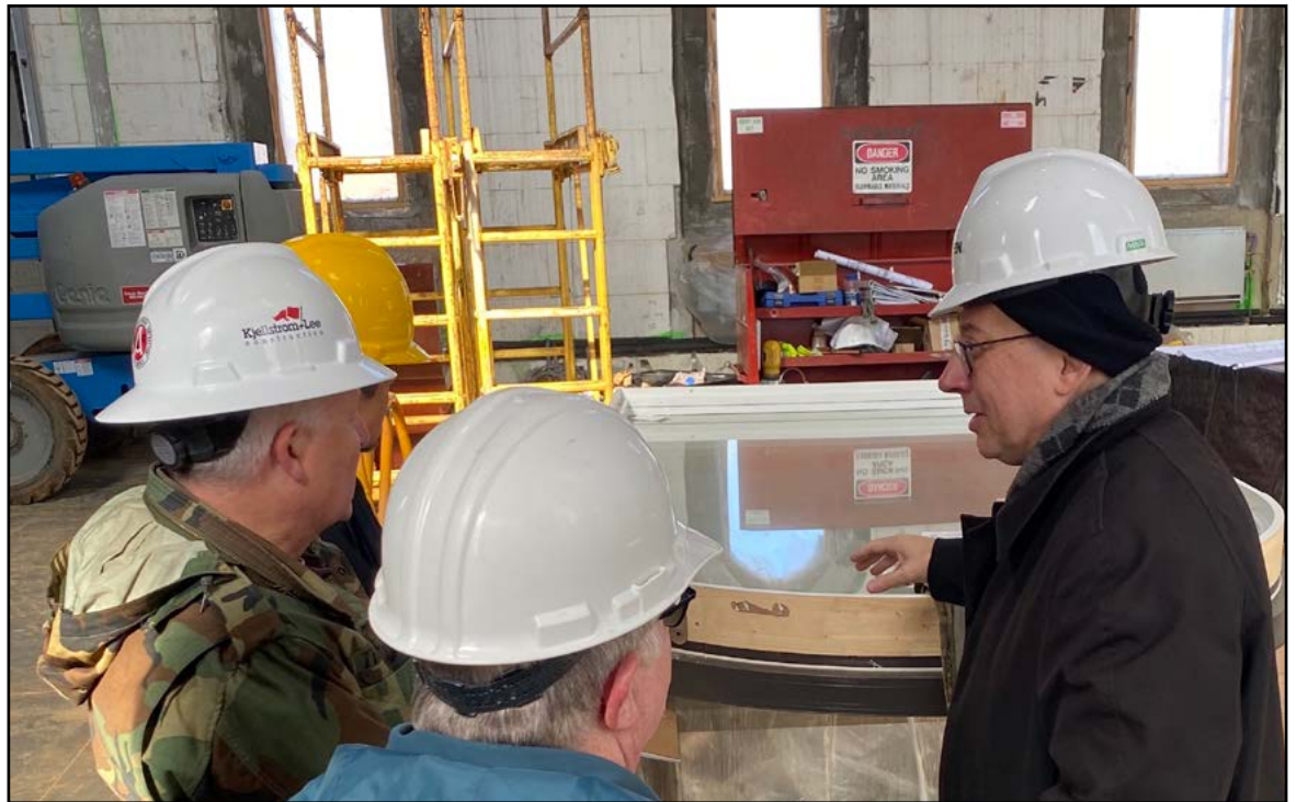
In February 2020, Bishop Barry C. Knestout visits the construction site of St. John the Evangelist, Waynesboro, a $12.5 million project supported by "Living Our Mission." The new church was dedicated on July 4, 2021. "Living Our Mission," a historic capital and endowment campaign designed for the benefit of parishes, schools and larger ministries, was launched in January 2014 with 14 pilot parishes and concluded active solicitation in 2016. (Submitted photo)
