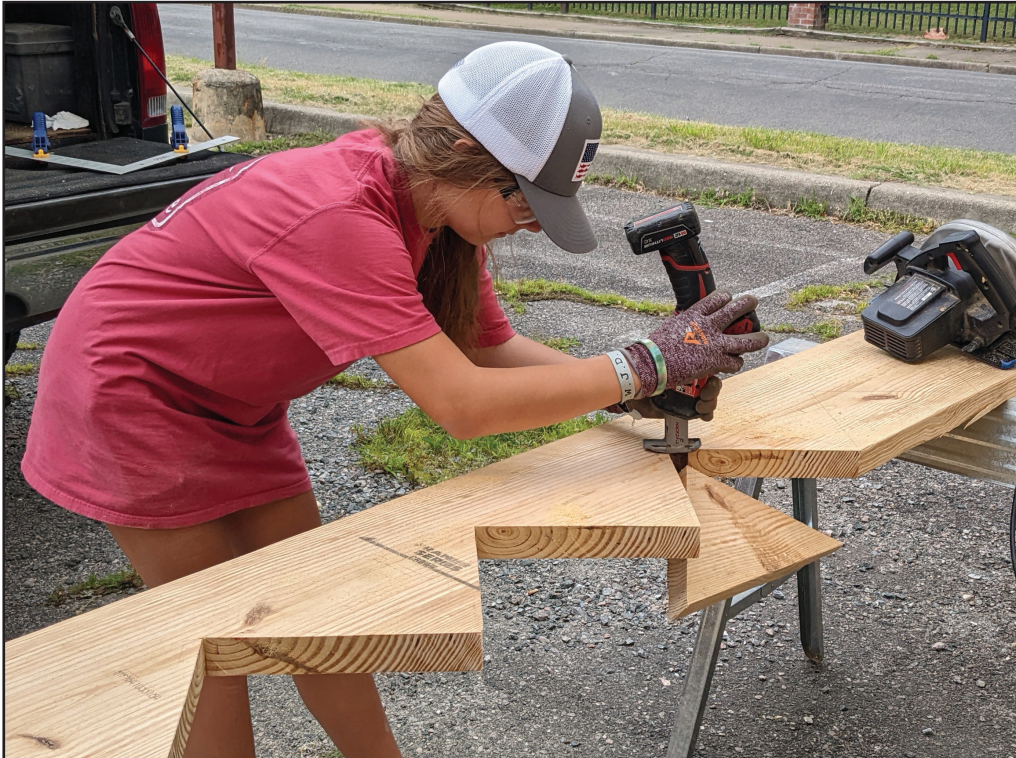
Natalie Yago, a member of St. Anthony Maronite Church, Glen Allen, helps to cut stringers for a staircase that she and her father, Chris Yago, built to replace stairs at Boaz & Ruth, a Richmond agency that aims to rebuild lives and communities through relations, jobs and economic revitalization. They were among the 150 volunteers from throughout the United States participating in the June 19-24 Catholic Heart Workcamp — one of Bon Secours Virginia Health System’s community wellness and revitalization initiatives in the Richmond area.
