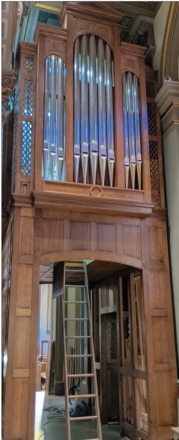
Pipes for the concert organ installed in the sanctuary at the Cathedral of the Sacred Heart, Richmond, are visible above one of the archways. The concert organ and a continuo organ are the first part of a $3.2 million project undertaken by the Cathedral of the Sacred Heart Foundation. (Photo provided)
