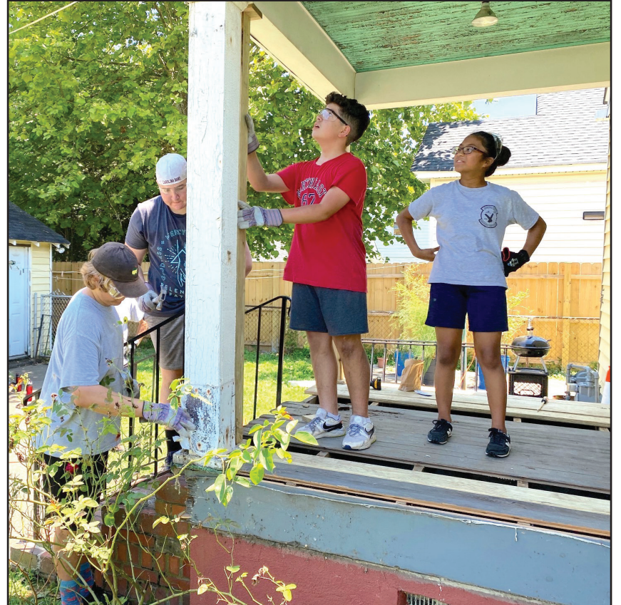
Members of a mission trip team at St. Jerome, Newport News, remove and replace a rotted porch column at a residence in their community on Friday, July 9. From left are Andrew Lombardi, Tommy Harrington, Leonardo Barreto and Hally Hallare. (Photo/Rich Arnold)
