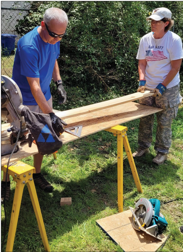
John Botelho and Bridget Rourke measure and cut a fascia board on Saturday, July 10, at one of the residences that received help from members of St. Jerome, Newport News, during the parish's local mission trip. (Photo/Delaine Botelho)
