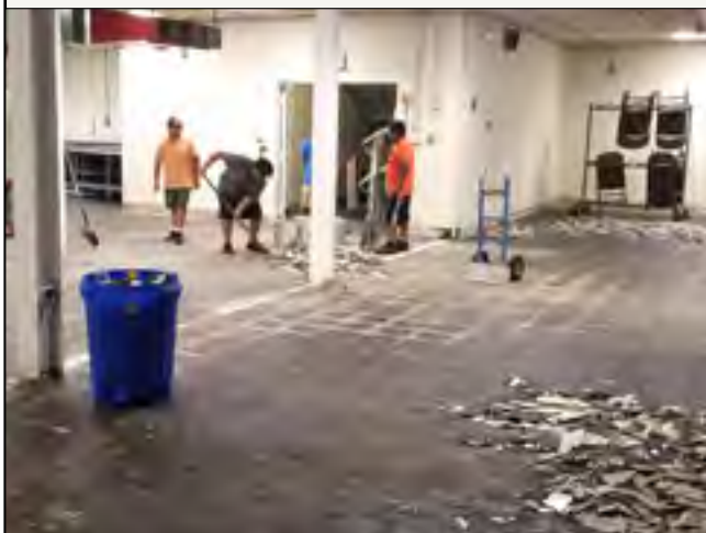
A crew of volunteers led by Carlos Martinez worked weekends and multiple nights over six months to gut and renovate the former school cafeteria into a St. James Parish gathering space. The group committed $20,000 in labor to the project. (Photo courtesy of St. James Parish)
